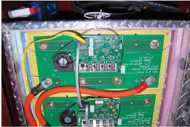
A battery management system protects its cell by shunting current around it when it is full.
